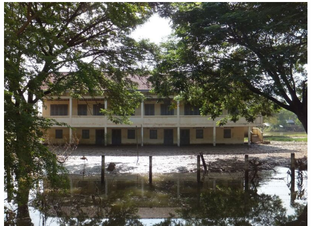
A rural school damaged by flooding in Battambang Province Cambodia in November 2011 (Credit: Carl Middleton)
