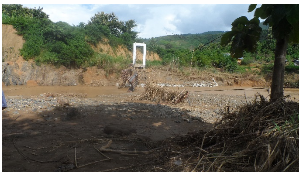
A bridge in Phonexay District, Luang Prabang province, Laos destroyed by a flood (Credit: Outhai Soukkyh)
