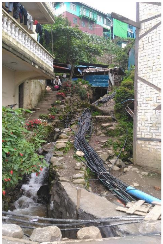
Tens of exposed and entangled pipes distribute water to individual houses (Credit: Carl Middleton)
